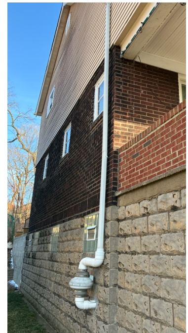
Exterior radon fan and stack Source: Christine Benner Dixon
